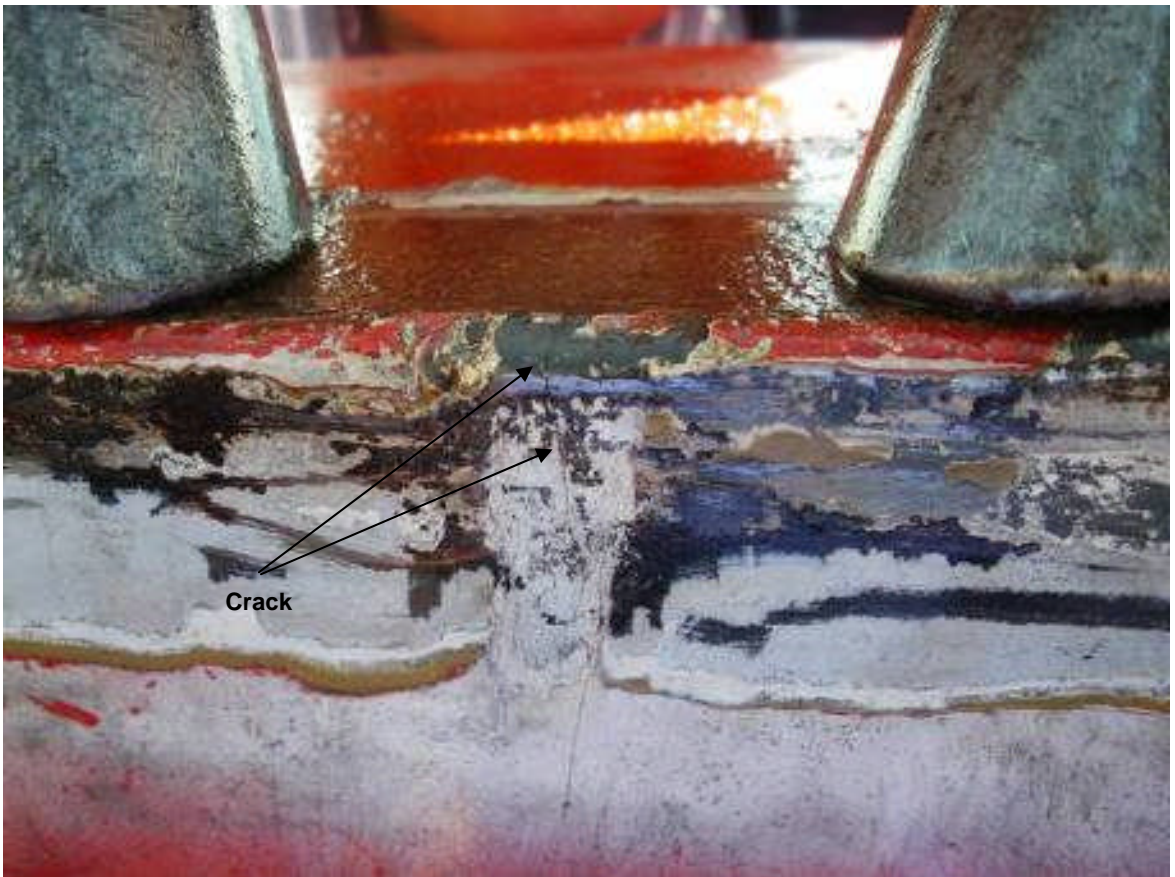
IMGP1610 – Crack Identified On-site using Magnetic Particle Inspection
